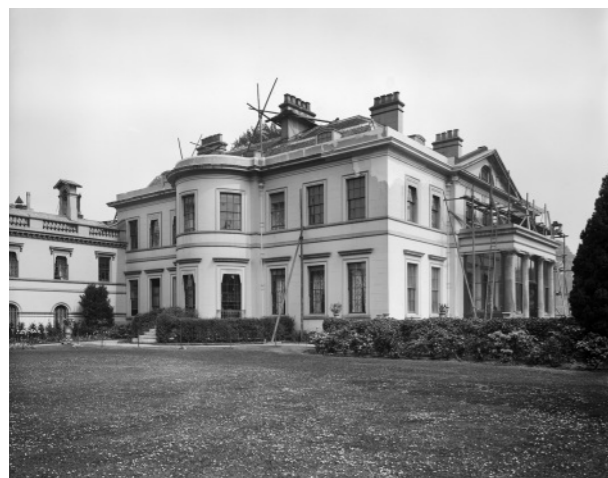
Fig. 1 Exterior view of Eastwick Park from the west, showing scaffolding erected on the roof and porch, 1910. Historic England Archive, BL20858. © Historic England Archive.
